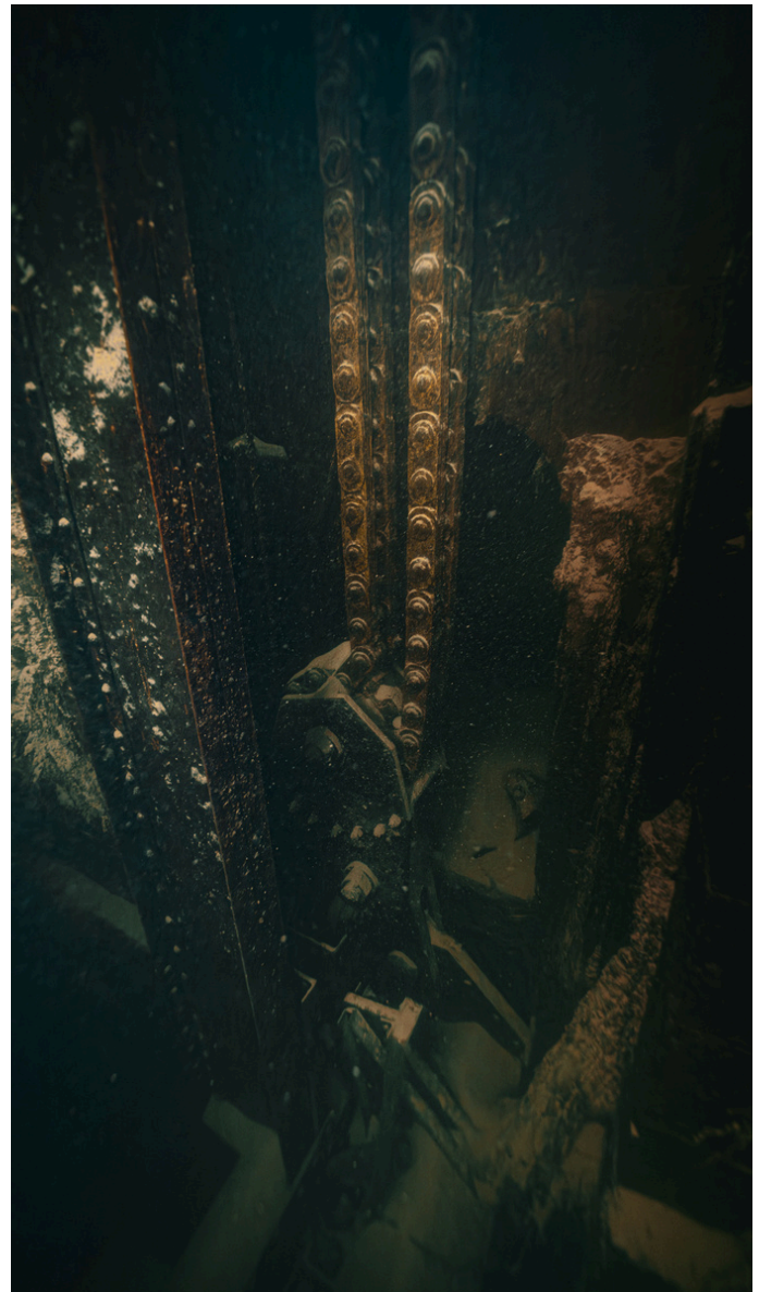
The lifting chains are still attached to the upper part of the valve, which they allowed to be lifted during maneuvers. © André PiedPalmé.
